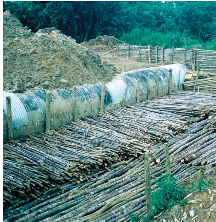
Fascine being laid on the Bau-Stass Road, in conjunction with a culvert, on particularly boggy ground, following a suggestion from Major John Stevens.
